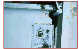
Fractured welded connections could lead to localized collapse. 1
