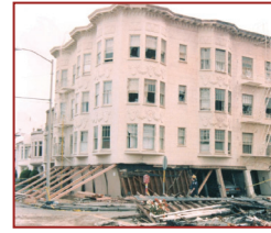
Nearly collapsed building first floor near Beach and Divisadero Streets in San Francisco during the Loma Prieta earthquake on Oct. 17, 1989. 4
