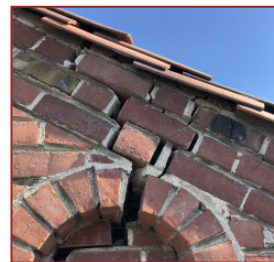
Wall cracking and permanent offsets are common in even moderate earthquakes.
