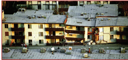
The Northridge Meadows apartment complex first floor collapsed during the M6.7 earthquake on Jan. 17, 1994. 3
