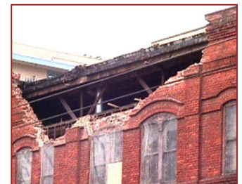
Lack of appropriate connection between roof and wall causing wall failure.
