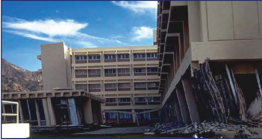
Image of heavily damaged non-ductile concrete building
