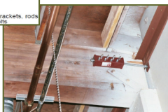
A typical retrofit with new wall anchors at roof-to-wall or roof-to-floor connections 2
