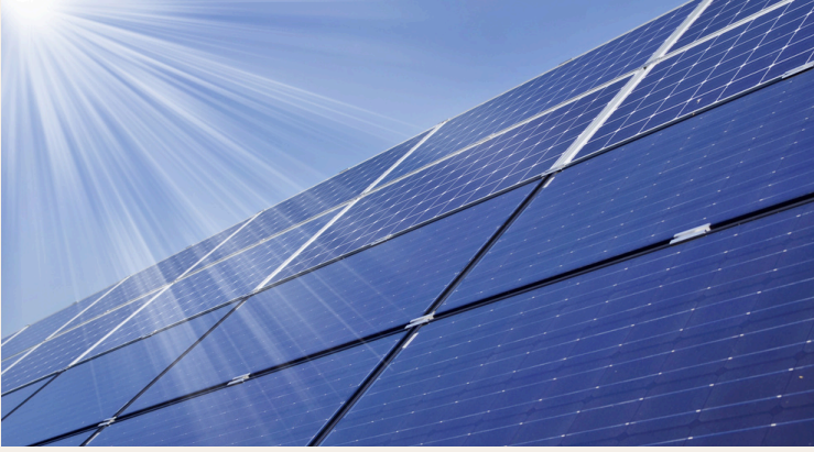
Solar panels at work: powering our world responsibly
