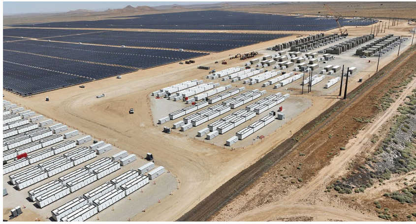
Solar PV and 3.3 GWh of battery Kern County, California
