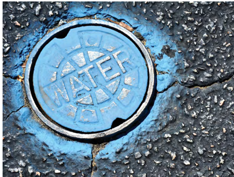
Blue water main on asphalt_StacieStauffSmith_shutterstock_2462608099
