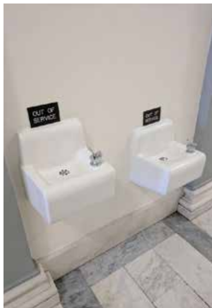
Drinking fountains in the Cannon Congressional Office Building. Marked “Out of Service” due to lead action level exceedances.
