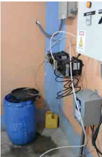
A typical chlorine dosing set-up in a well house. The peristaltic pumps draw the chlorine solution out of the blue tank and dose it into the reservoir where it achieves proper contact time.
