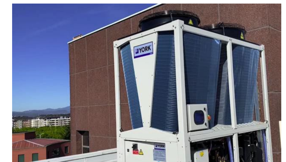
Leon, Spain Ambulatory Center, YORK Distribution
