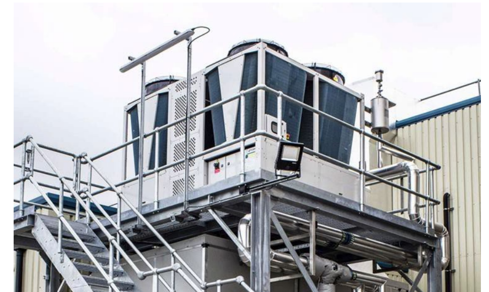
Morrisons Wakefiled Pitta Line, Beswick Refrigeration, UK
