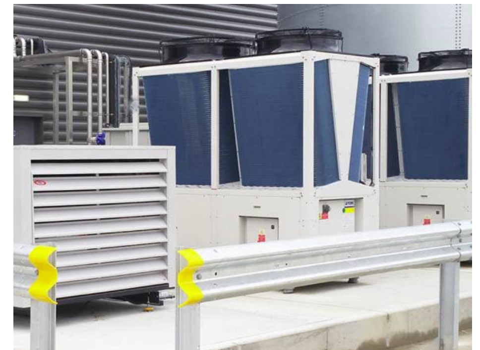
Biotechnology Coldroom, Beswick Refrigeration, UK
