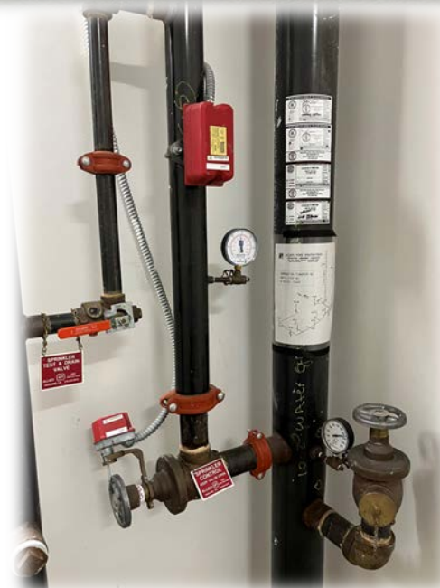
Sprinkler Control Valve
