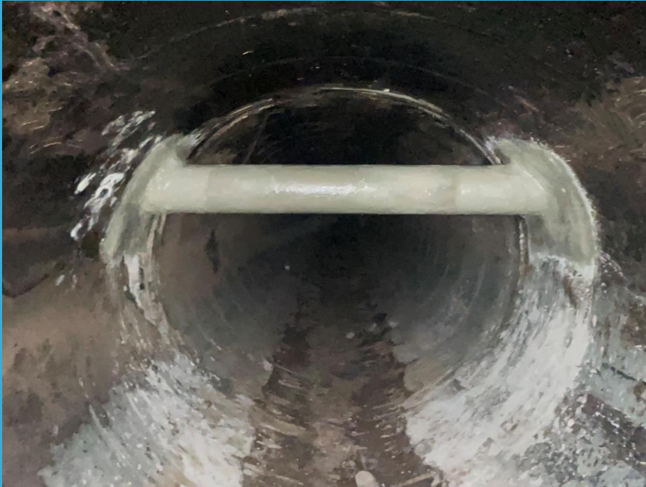
FRP (Fiber Reinforced Polymer for exterior protection of sewer crossing storm drains)
